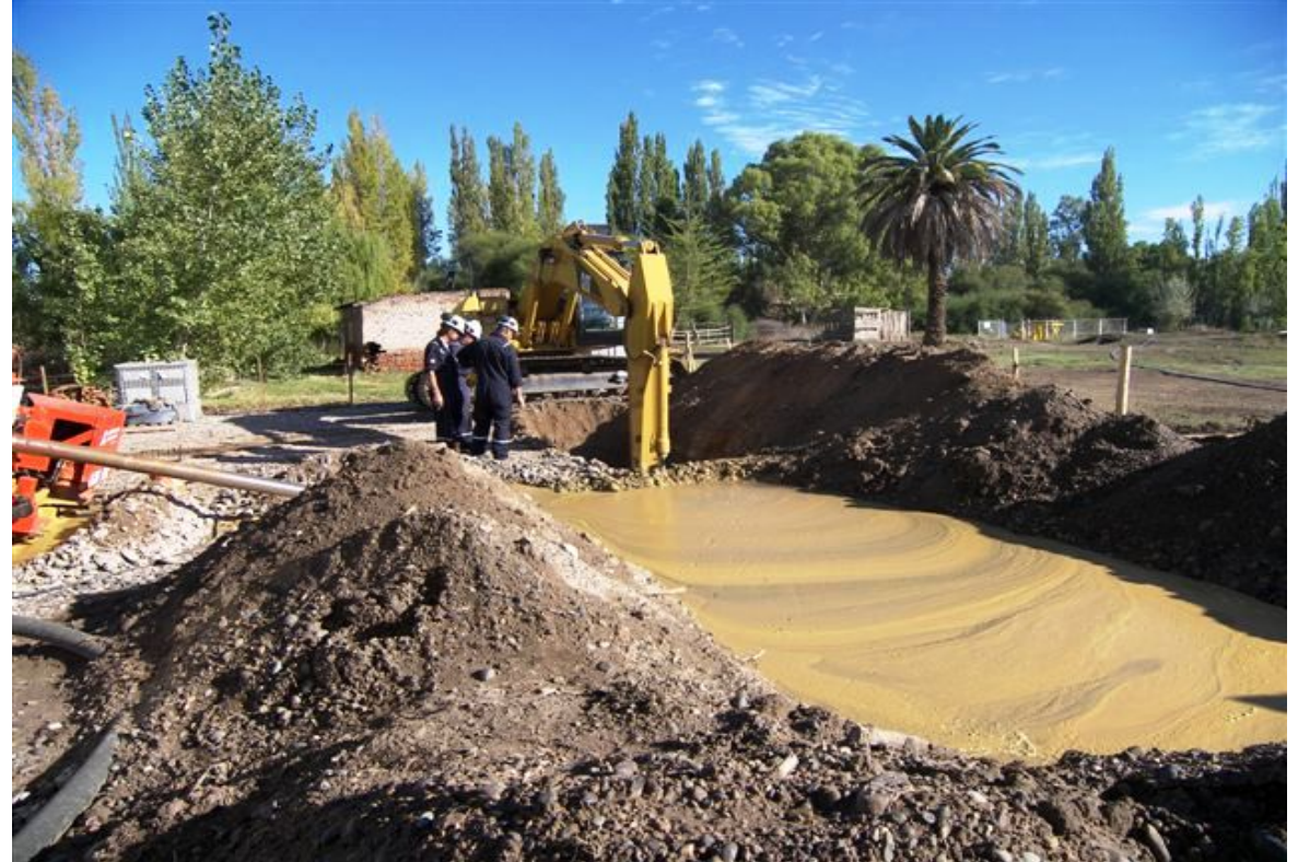
HDD project in Argentina in “pump and dump” mode creating 3500 m3 of waste for each project
