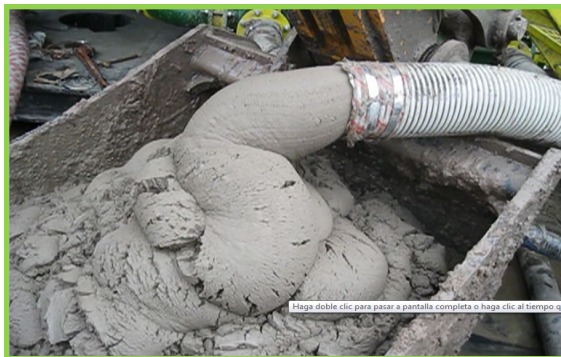
QDNT Solids Discharge
